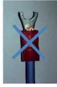
Terminal has been cut.
