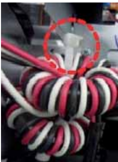
Binds a Comp wire-core to Bracket beam control box using large size Cable-Tie(350mm).
